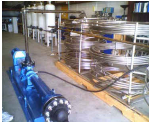
Figure 6: Scavenger system in the beginning
