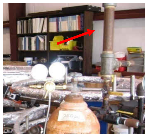
Figure 10: Scavenger injection vessel
