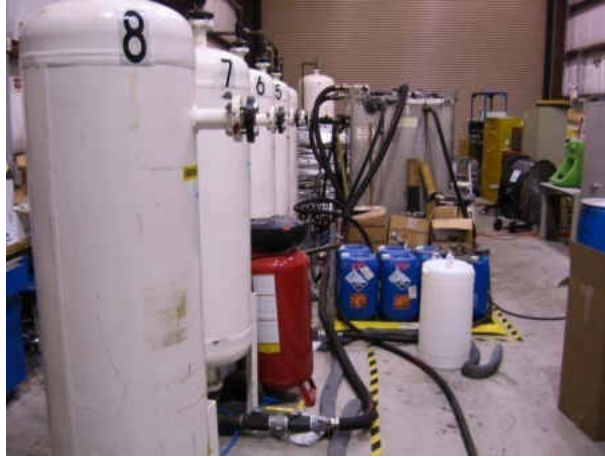
Figure 13: Scrubbing system, Tanks 6, 7, 8.
